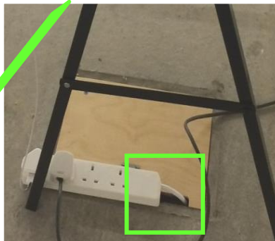
The cable has been fed into the inside of the floor box minimizing the amount of cable exposed.
